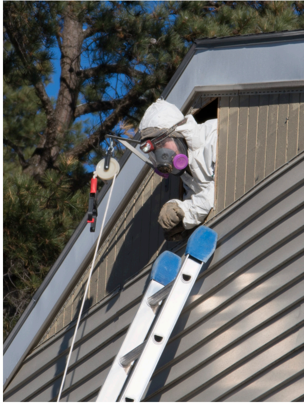
An insulation contractor works in the attic space of Royal Concord Gardens, adding loose fill insulation.
